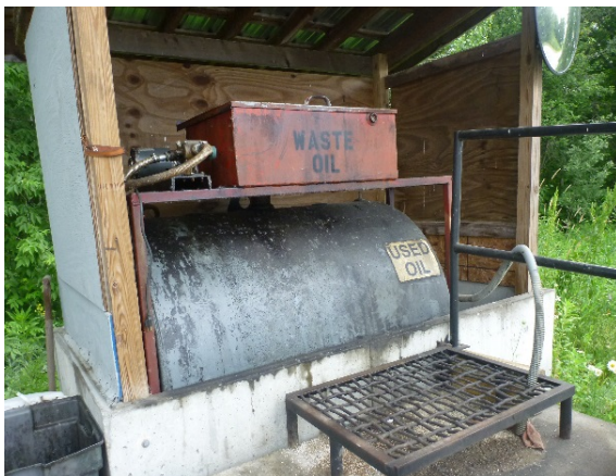
Proper secondary containment for an aboveground storage tank holding used oil outdoors
