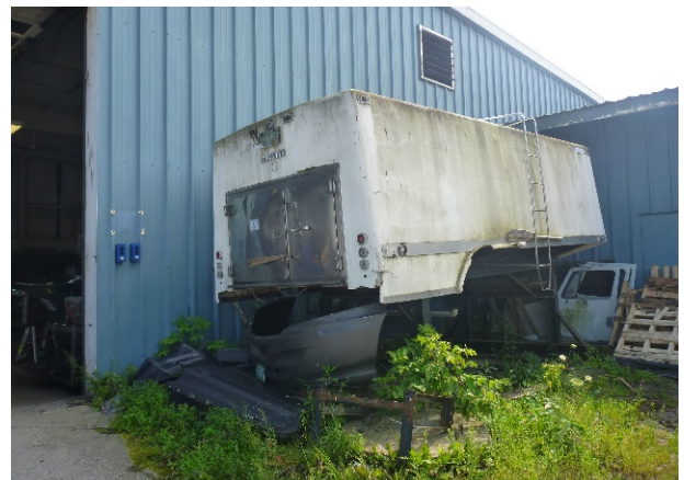
Improper secondary containment for aboveground storage of used oil outdoors - single-walled, unlabeled tank trailer
