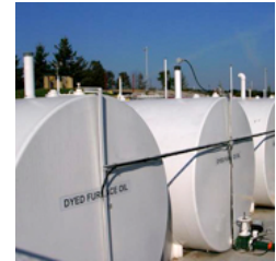
Tanks of heating oil ( discountheatingoil.com )
